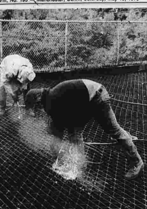
Repairs Under Way. Repair work has started on the Park Street Bridge. Eugene Warner Jr., left, and Arthur Balch, both of Black & Warner.
